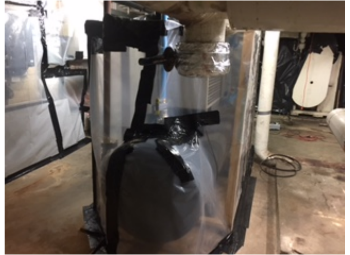
Encapsulation of boiler
