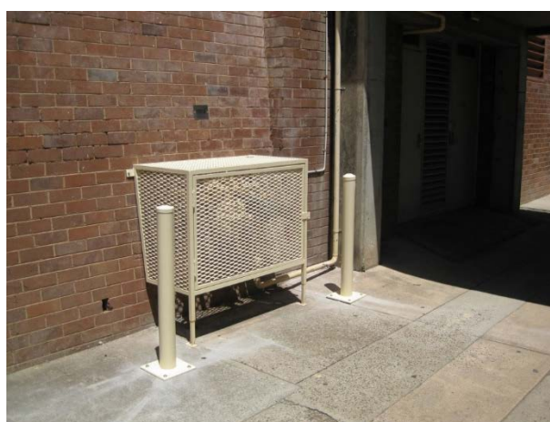
Figure.1: Typical ANU gas meter enclosure
