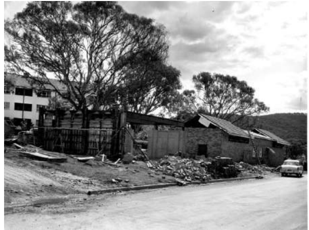
Figure 2.20 Molly Huxley Building under construction 1963. Note the old PABX building (disjointed roofline mid-way along structure) being incorporated into the new structure. (Source: ANU Archives 2015)
