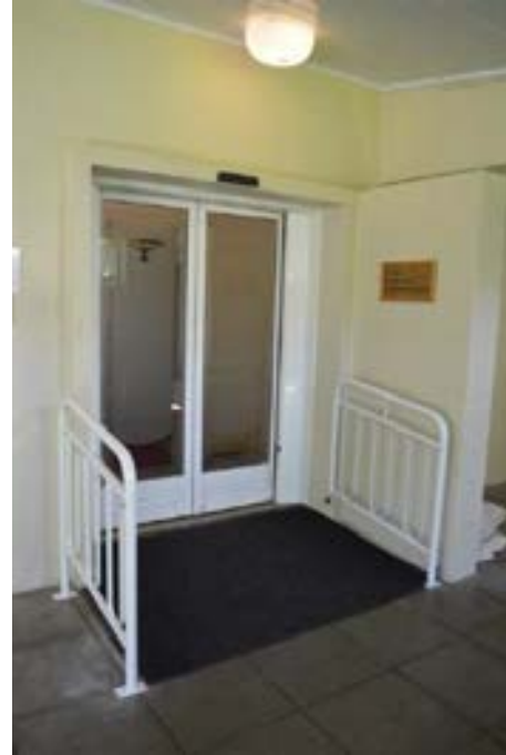
Figure 3.51 Aluminium-framed automatic sliding doors to the entrance portico between the hall foyer and the Common Room. (Source: GML 2015)
