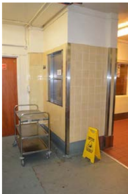
Figure 3.124 Dumb waiter in the kitchen. (Source: GML 2015)
