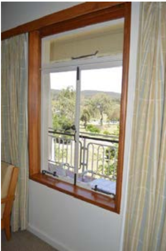
Figure 3.86 Original timber and steel window framing in the accommodation wing. (Source: GML 2015)
