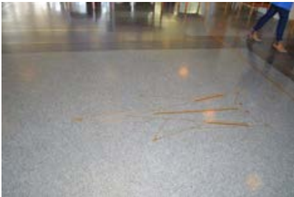
Figure 3.18 Entrance foyer showing brass inlay terrazzo floor designed by Frank Hinder. (Source: GML 2015)
