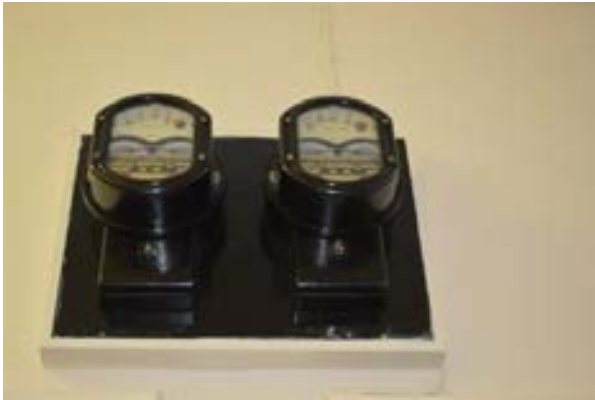
Figure 3.108 Original electricity meters in the Western Annex. (Source: GML 2015)
