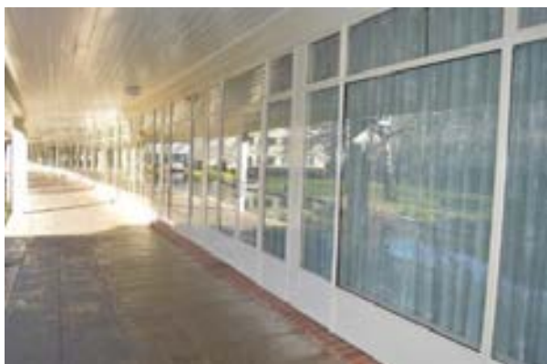
Figure 3.43 Terrace showing the glazing and steel-framed windows and doors of the Common Room. (Source: GML 2015)
