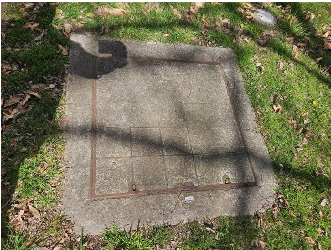
Figure 4: Neutralising Buffer Tanks
