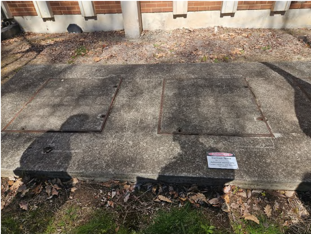
Figure 3: Neutralising Buffer Tanks
