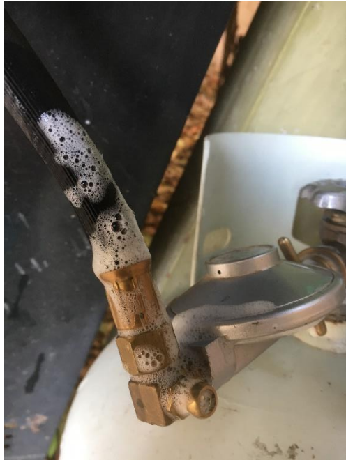
Gas hose and fittings
